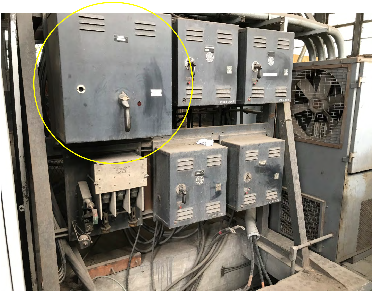
Broadway Marine Terminal D Building Substation Existing 480 V Switchgear
