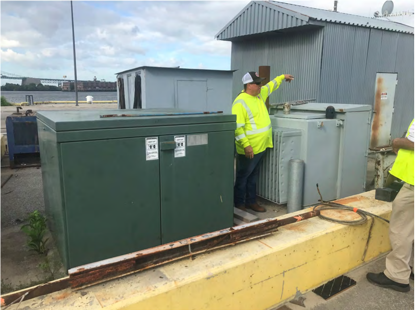
Pier 1 Outdoor Equipment 4,160 V Switch Cabinet on Left 4,160 V Transformer on Right
